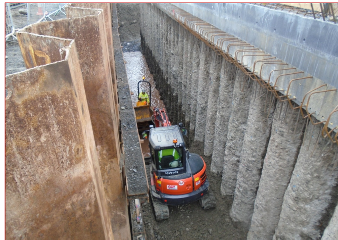
The excellent line of the wall demonstrated our ability to drill accurately in strong materials.
